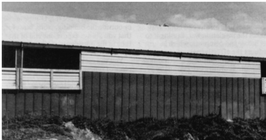
Figure 5.—Openings may be moving enough air, but it appears that inlet distribution is not uniform.
