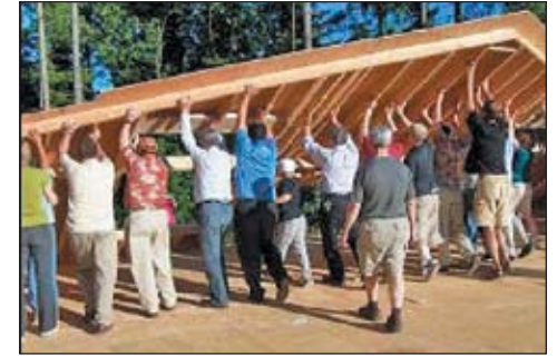
Chamber of commerce members from Oregon City, North Clackamas and West Linn came out last June to help raise a wall for the new classroom being built at Hopkins.
