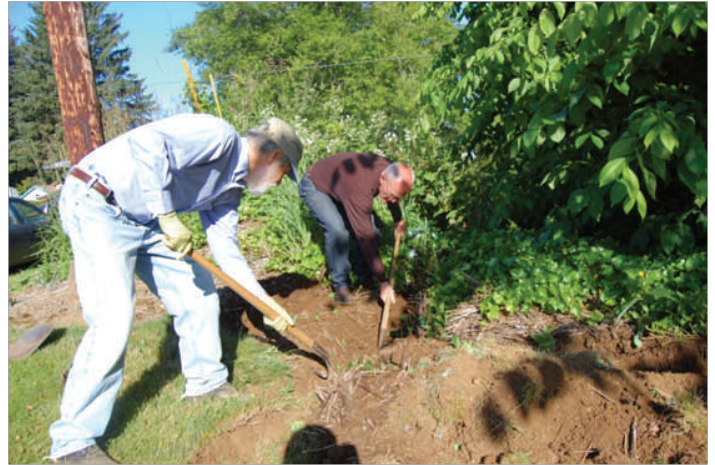
Above: Volunteers Mick Dressler and Gary Albright put their backs into installing a silt fence along Patterson Creek in advance of building Bay City's first rain garden.
