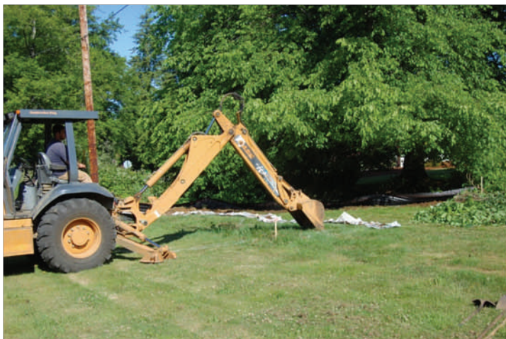
Above: A City of Bay City backhoe operator carefully digs out the basin for the rain garden.
