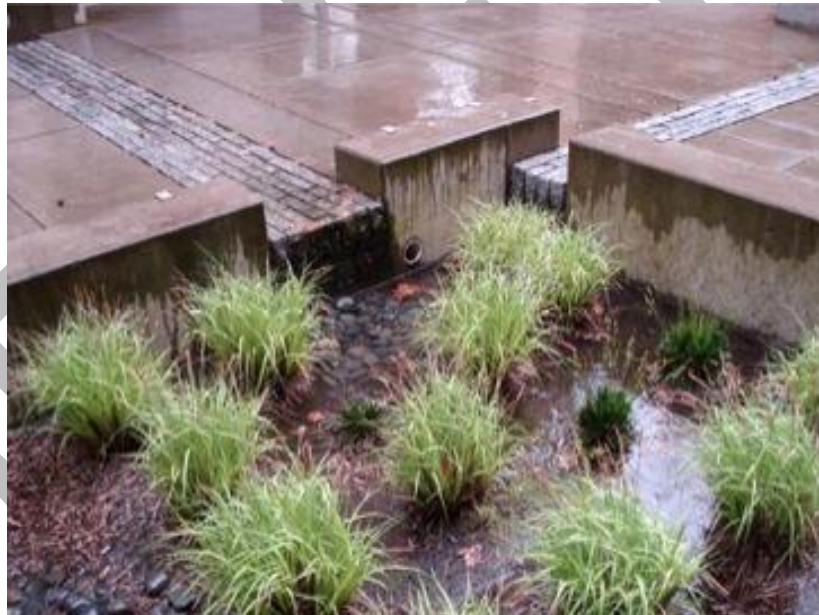
Figure 1 Stormwater Planter at Epler Hall on the Portland State University Campus, Portland, OR (PSMM 2008)
