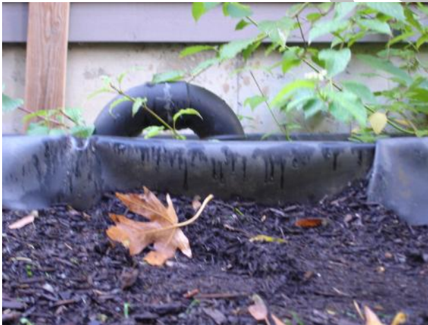
Figure 5 Improperly installed U-shaped overflow
