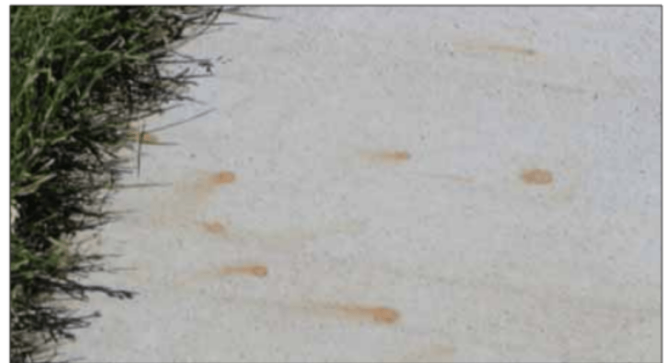
Figure 4. Brown rust stains where iron contacted concrete and then was watered in.
