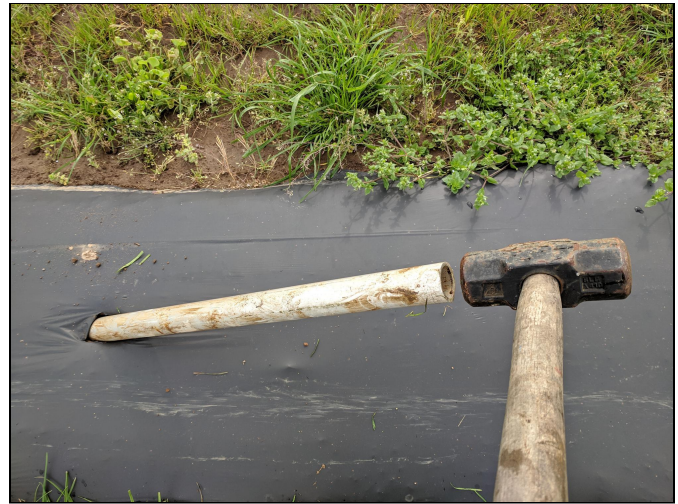
Figure 4. Insert metal pipe at the ends of the tunnels at a 45-degree angle to keep the plastic secure and taut.
