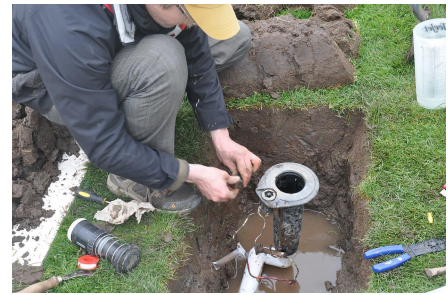
Figure 7. Automatic control irrigation systems typically have wiring to each irrigation head or a block of irrigation heads to provide more precise irrigation.
