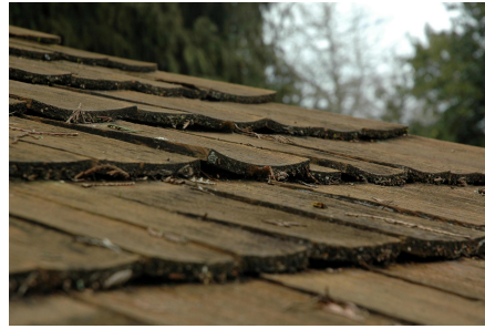
Figure 3b. Cupping and shrinkage of cedar shingles.
