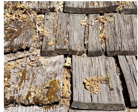
Figure 3c. Splitting and shrinkage of cedar shingles.
