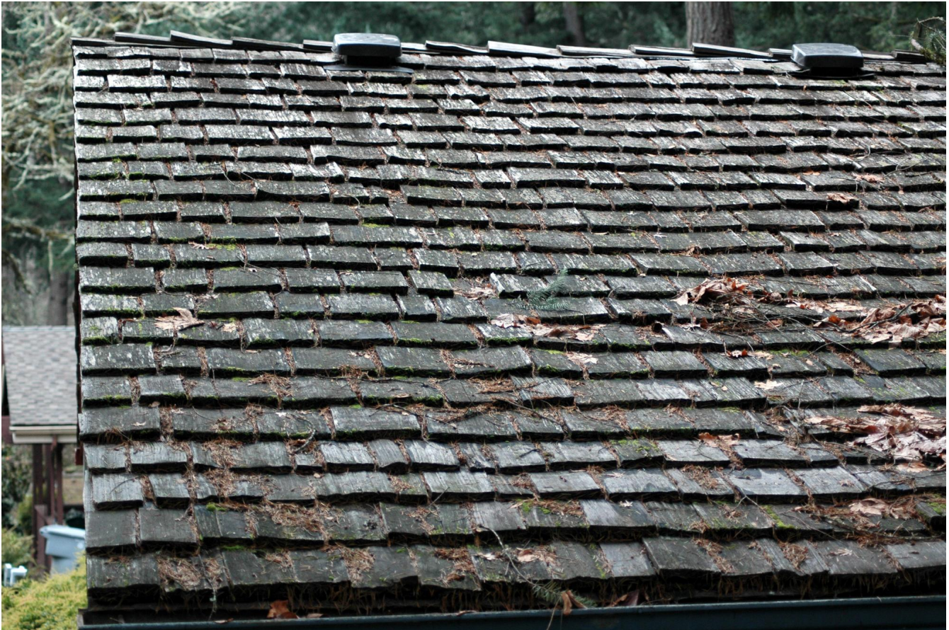
Figure 6. Remove all leaf litter, conifer needles and debris that accumulate between the shingles and shakes and in the valleys. It's best to do this before the wet season begins.
