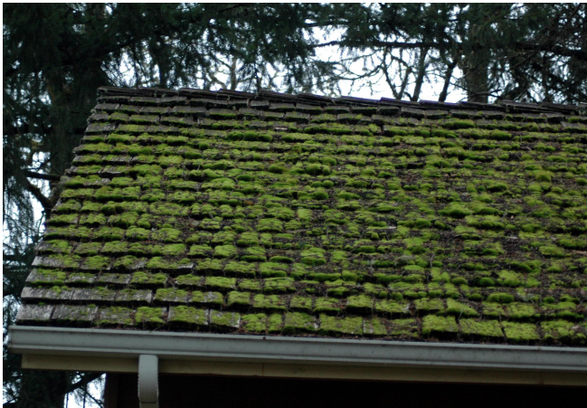
Figure 5a. Moss builds up quickly when roofs are shaded by trees.
