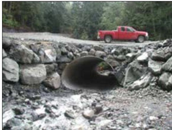
Figure 4.10. Dipped rock fills result in stable road prisms at stream crossings. Note the large-arch culvert, heavy-rock armorings, and minimal fill over the culvert.
