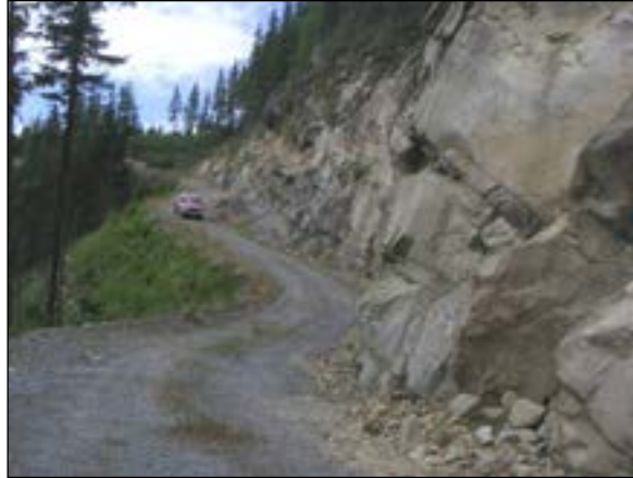
Figure 4.9. Full-bench construction ensures that no unstable fill material is placed along the outside edge of the road and that hill-slopes below the road remain at their natural angle of repose.
