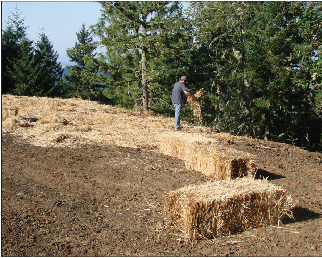
A pond builder spreads out straw along the downslope of the excavation site where the pond will be. Straw makes an excellent weed deterrent and is an environmentally sound way to control both weeds and erosion. The straw will also attract a variety of wildlife.
