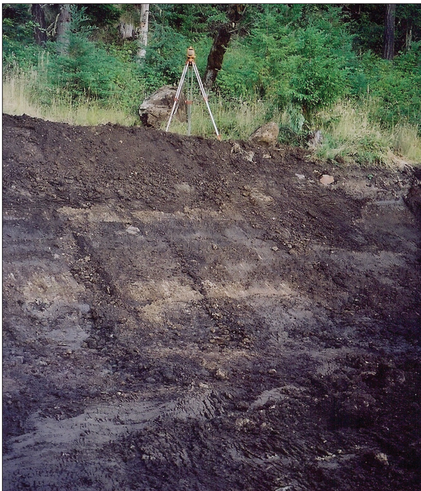
A laser level should be located where it can remain out of the way throughout the construction project.
