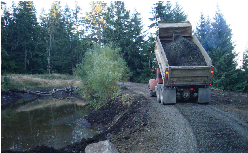
A dump truck can be used to remove soil from a pond site and then used to deliver and spread rock along the road.
