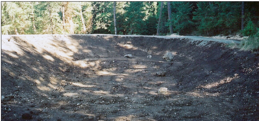
A completed pond sits with the first lift of rock on top of the dam.
