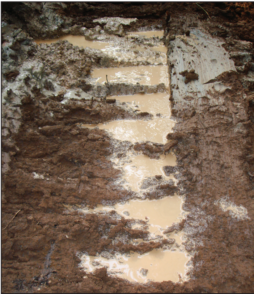
When initial excavation reveals heavy clay soils and water seepage, you may have found the ideal location for a pond.
