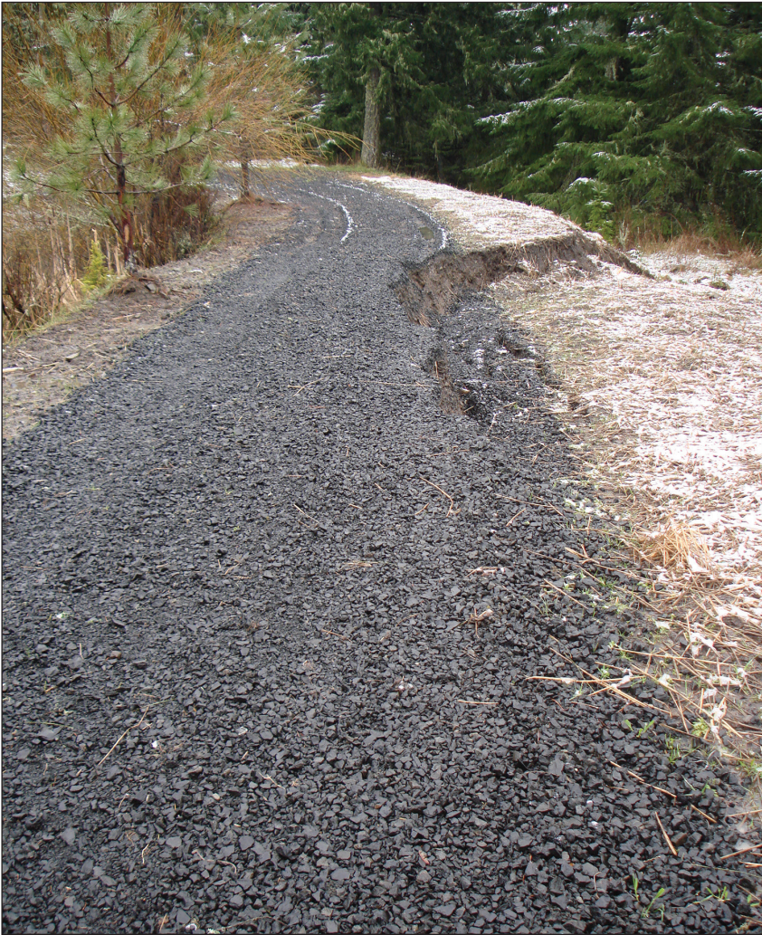
Soil movement caused by ponds can damage poorly placed roads, leading to costly repairs and environmental damage.
