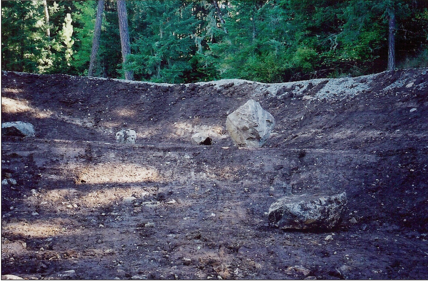
This completed pond has incorporated multiple water levels and rocks to serve as habitat for fish.
