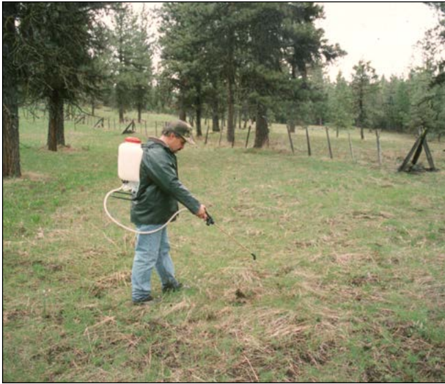
Figure 9. Backpack sprayers, for spot sprays or broadcast applications, are an effective, cost-effective way to apply water-based herbicides. Sites with gentle terrain and little slash or other obstacles are good candidates for this method.
