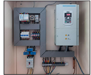
Figure 7. An electrical control panel with variable frequency drive, or VFD, used to regulate pump operation and system pressure.
