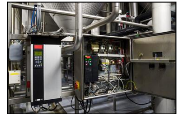
Figure 8. Variable frequency drive, or VFD, system used to adjust motor speed for improved irrigation efficiency and energy savings.
