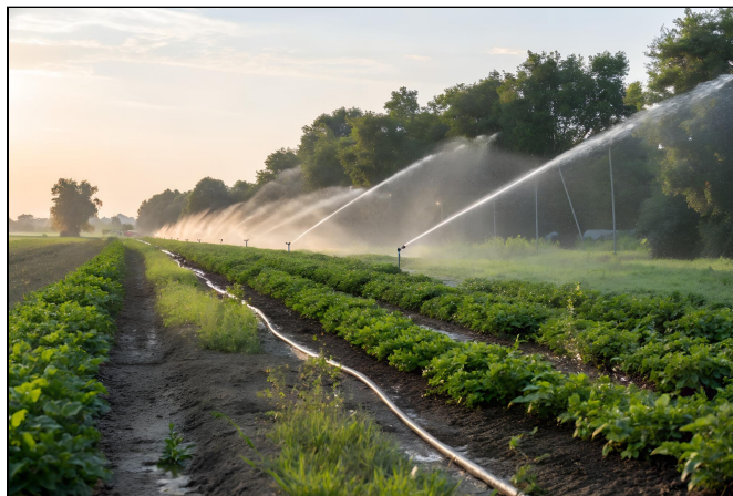
Figure 9. Solid set sprinkler irrigation system operating in a vegetable field, showing permanently installed laterals and evenly spaced sprinklers used for uniform water application.
