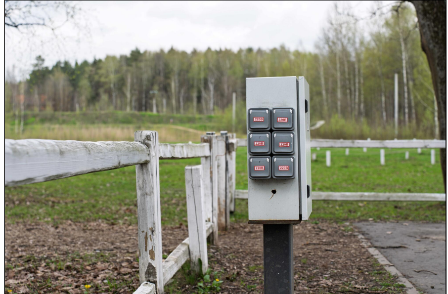
Figure 3B. An electrical service panel in an irrigation pumping system.
