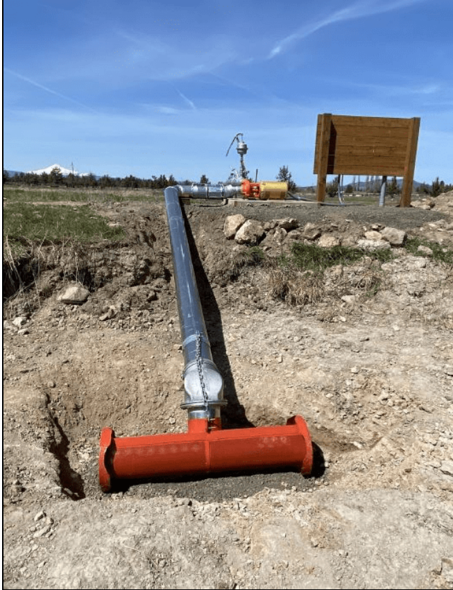
Figure 2A. A pump intake filter system. Regular inspection of these components helps ensure adequate water flow and reliable operation of the irrigation system.
