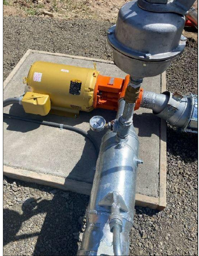
Figure 2B. An irrigation pump with an electric motor assembly.
