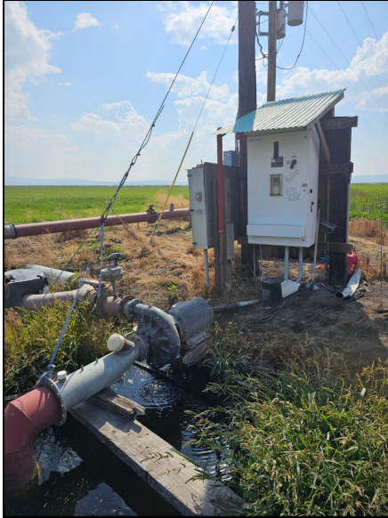
Figure 3A. Irrigation electrical components include variable frequency drive controls used in irrigation pumping systems.
