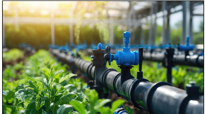
Figure 4B. A properly maintained pipeline. Regular inspection helps detect leaks and maintain system pressure and efficiency.
