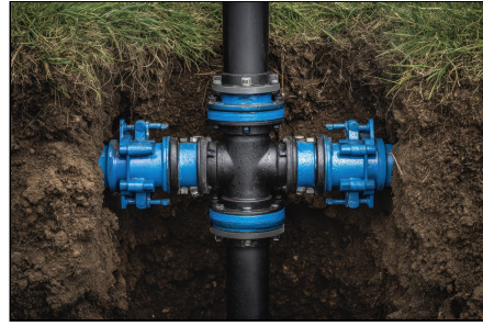
Figure 10B. An underground pipeline manifold distributes water to multiple lateral lines.
