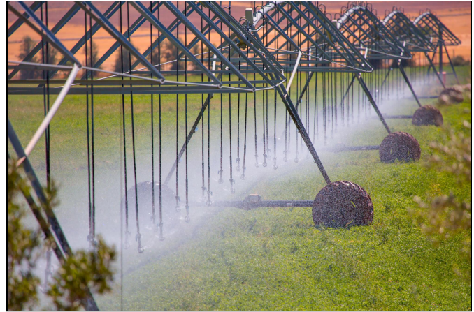
Figure 13B. A lateral-move irrigation system moves in a straight line across a field.
