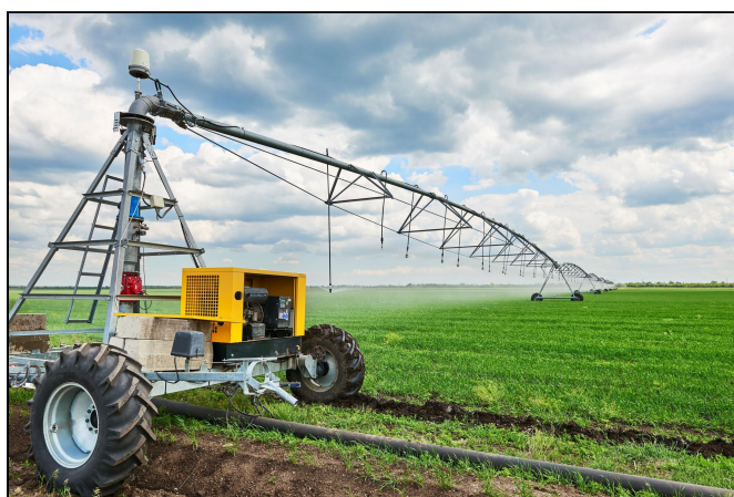
Figure 14B. Inspection of the pivot tower, drive system and control components ensure proper mechanical and electrical function.
