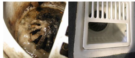
The drain on the left needs to be cleaned, the drain on the right has been maintained in excellent working order.
